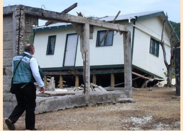
An aid worker conducting a needs assessment inspects tsunami damaged housing in Tonga.
